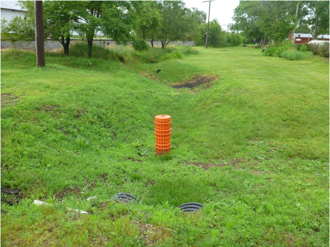
Figure 2.9. View near the intersection of 3 rd Street and the railroad, looking northeast. Twin 18-in corrugated plastic culverts convey ditch flow under 3 rd street. An orange riser is connected to the 18-in pipe that drains the pond.
