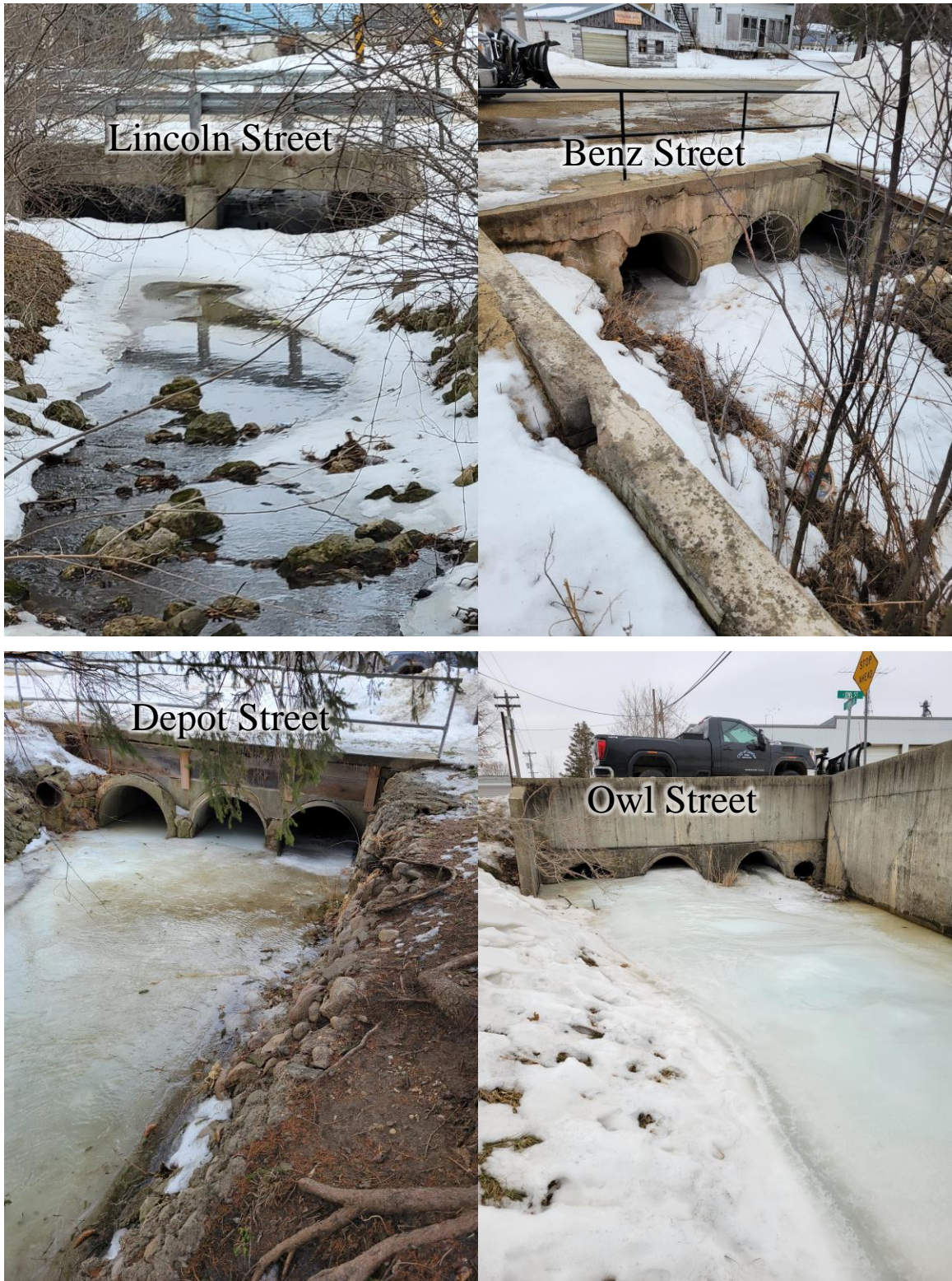
Figure 13. Photographs of culvert crossings that would benefit from upgrades in Lawler, Iowa.
