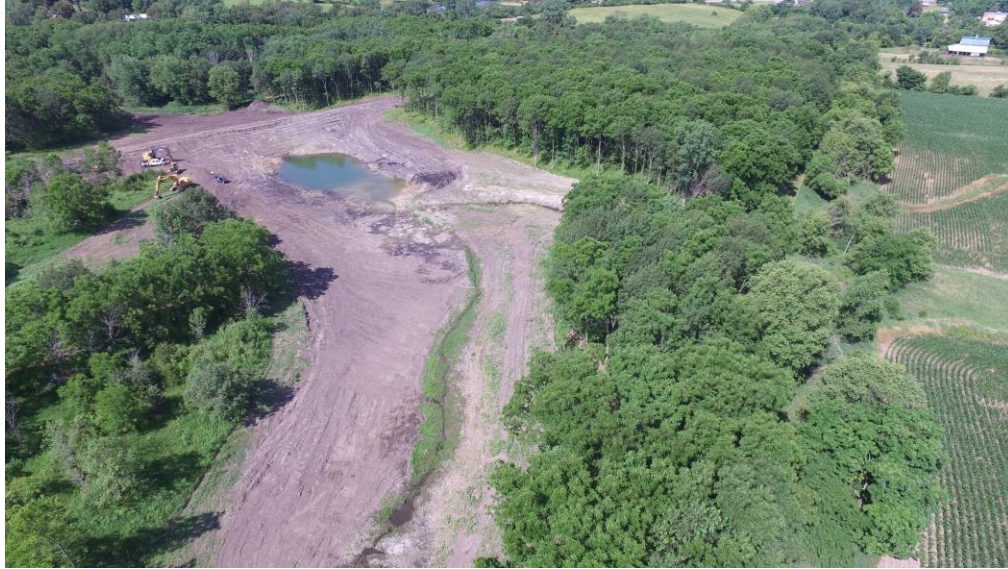
Figure 1-3. Flood mitigation pond and fringe wetland (CC-015 Sippy) constructed as part of the IWA in the Middle Clear Creek watershed, a sub-watershed of Clear Creek.
