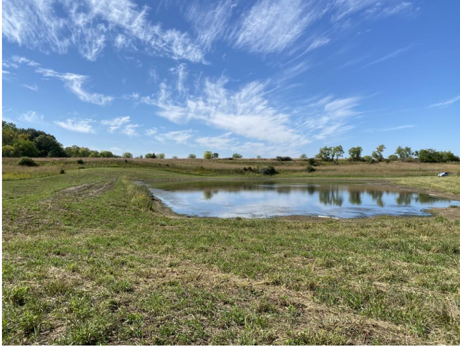
Figure 1-4: Flood mitigation pond (CC-010 Asumussen) constructed as part of the IWA in the Middle Clear Creek watershed, a sub-watershed of Clear Creek.
