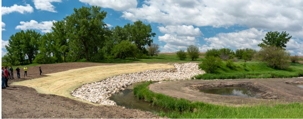
Figure 1-3: Flood mitigation oxbow and stream stabilization project (NR-001 Rob Smith) constructed as part of the IWA in the Outlet Creek HUC12, a sub-watershed of the North Raccoon HUC8.
